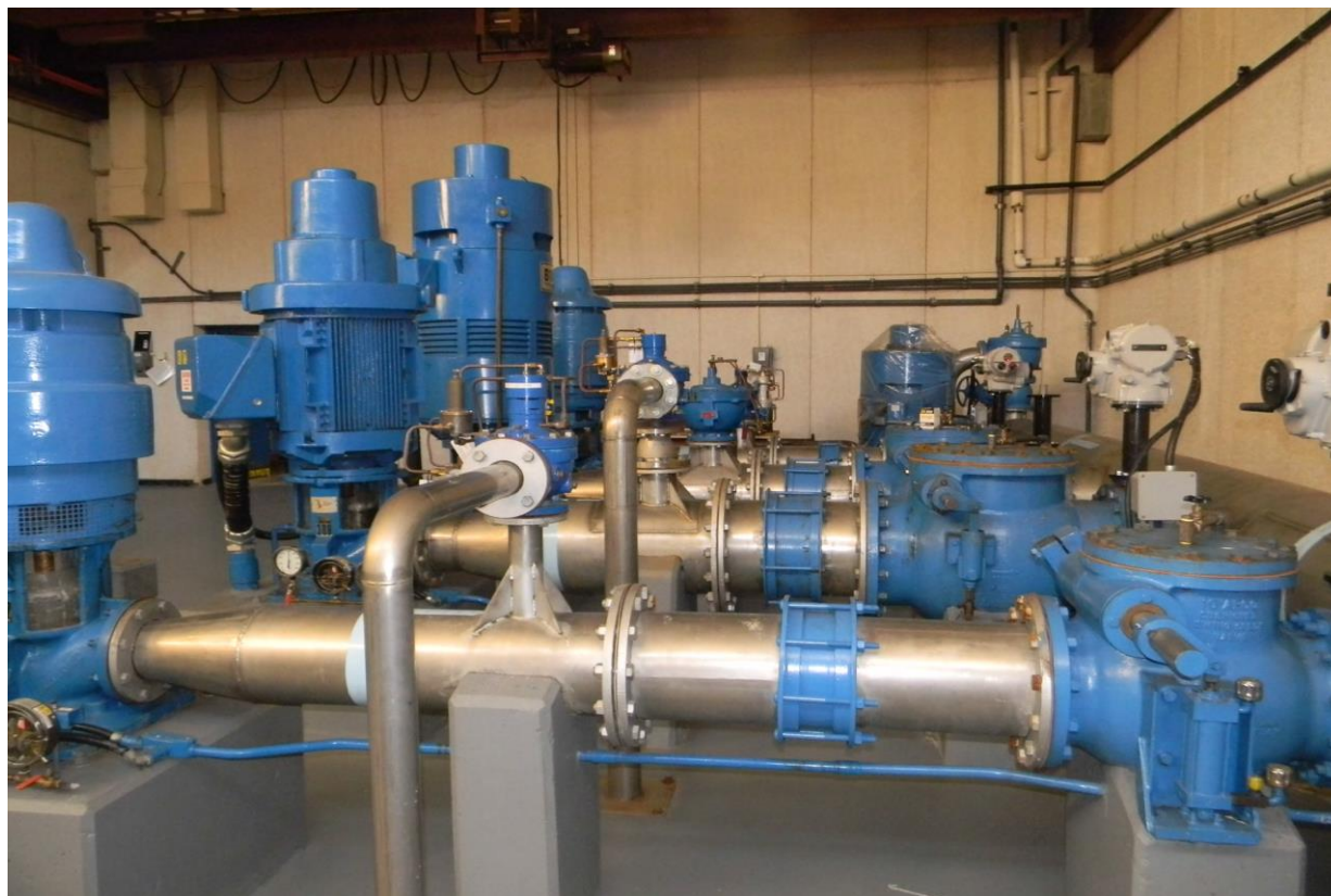
Figure 2 – Water Treatment Plant (Low Lift Pumps)
